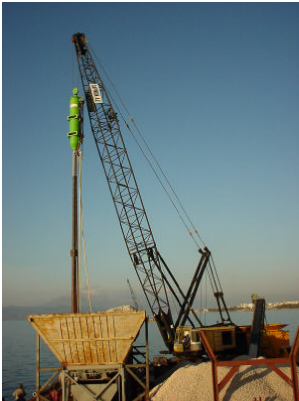
Fig. 6: Gravel silo and conveyor belt (front), crane with 24 m long Marine Gravel Pump unit (back)
