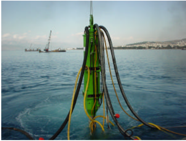
Fig.5: Double lock batching tank with Schnorchel hose (left) and two gravel hoses (right)
